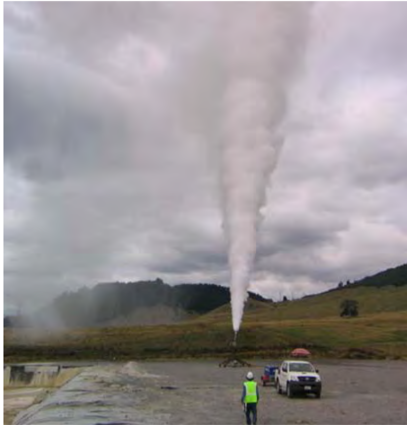
TH-12 vertical discharge
